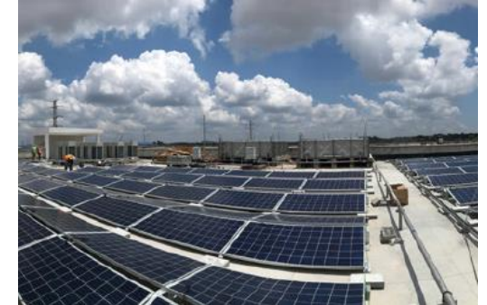
Solar plant in Gebeng
